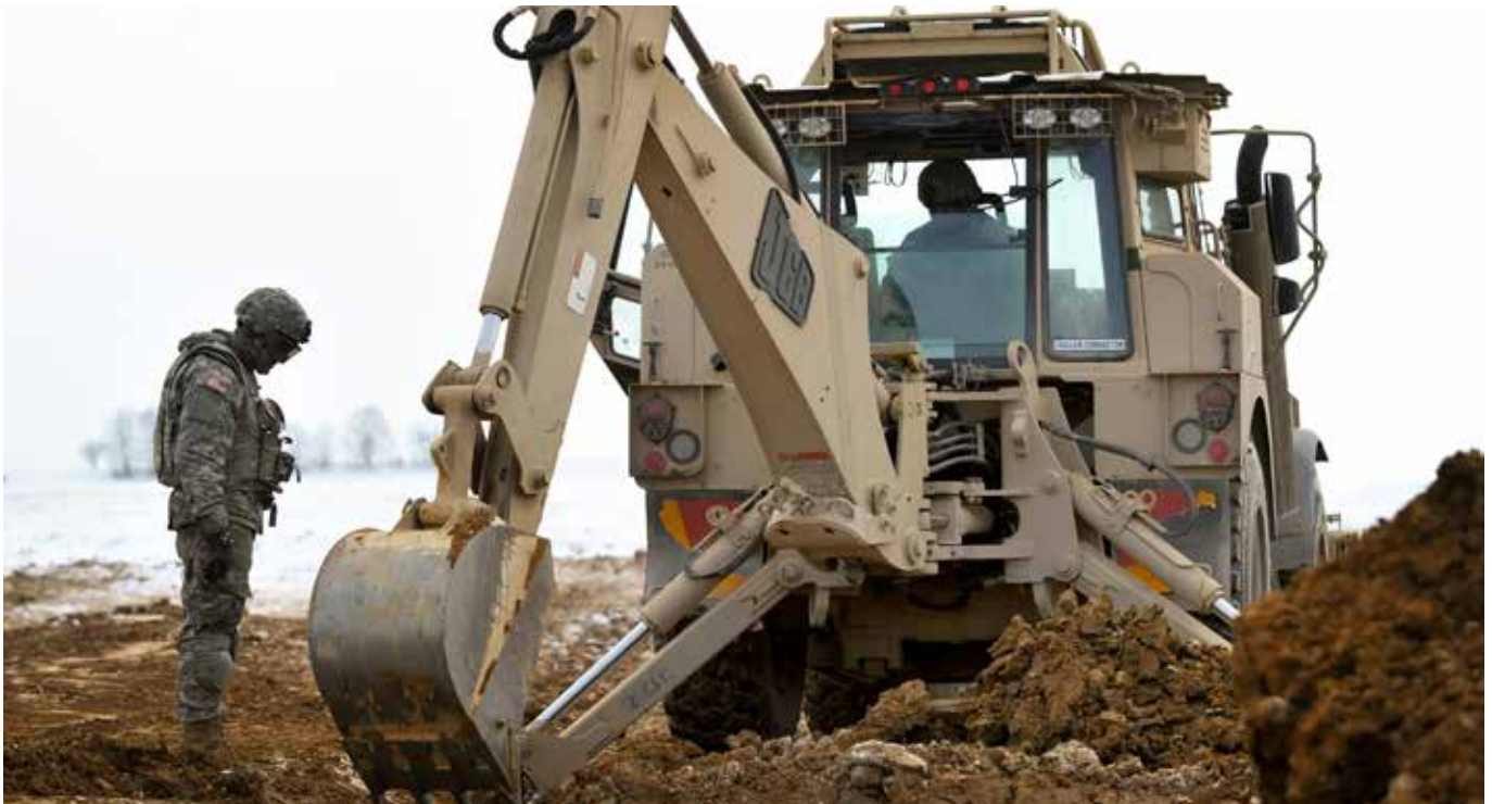
Engineers from the 2nd Cavalry Regiment perform dig site operations at the Grafenwoehr Training Area in Grafenwoehr, Germany, on Feb. 14, 2013. (Photo by Markus Rauchenberger)
